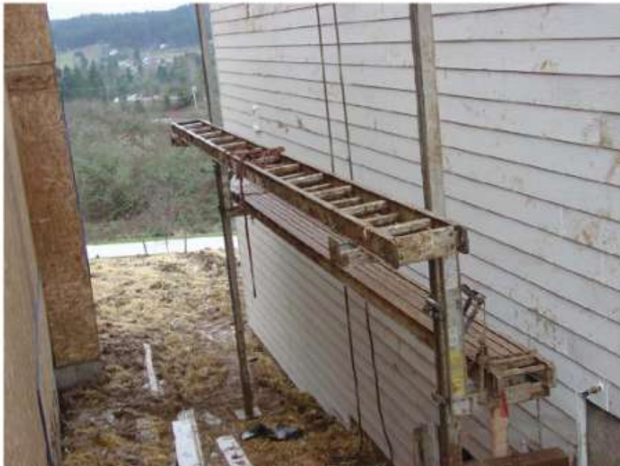
Pump Jack Scaffolds will normally have a work bench that can act as a top rail if it is 38 to 45 inches. Don't forget a midrail and guarding the ends – both are missing in this picture.
